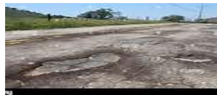
FAULTY ROAD SURFACE?
