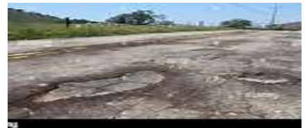
FAULTY ROAD SURFACE?
